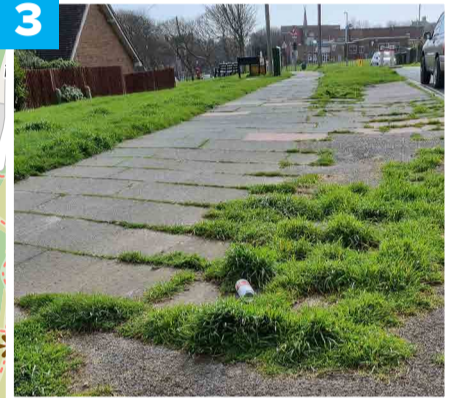
3 Labour banned the use of weedkiller - without putting any alternatives in place. Pavements are blocked and hazardous for the elderly.
