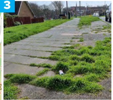
3 Labour banned the use of weedkiller - without putting any alternatives in place. Pavements are blocked and hazardous for the elderly.
